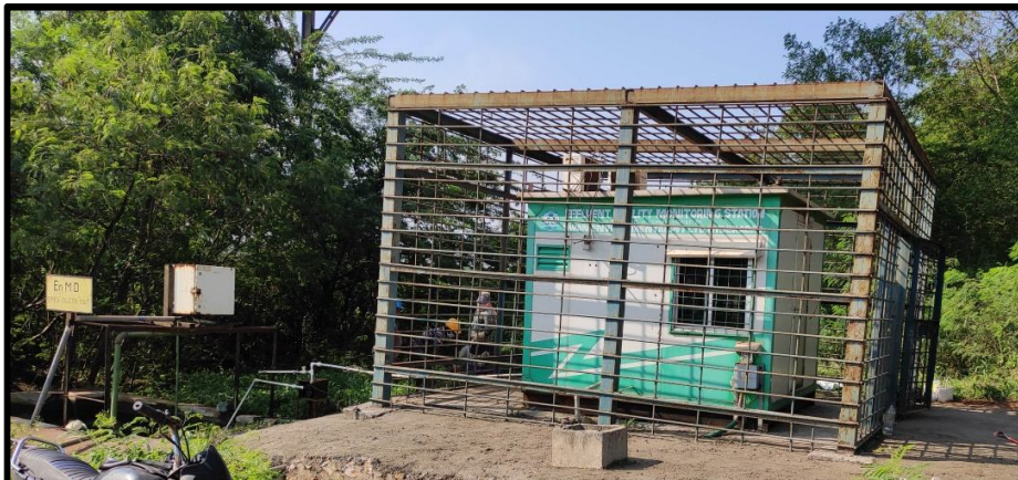
Continuous Effluent Monitoring System installed at ETP
